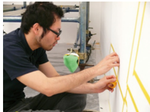
Segments of the wall are masked with tape and the area inside painted.
